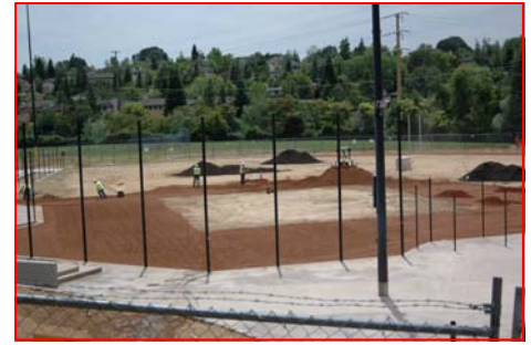
Jeff Mitchell Field construction is proceeding. The Grand Opening is scheduled August 29.
